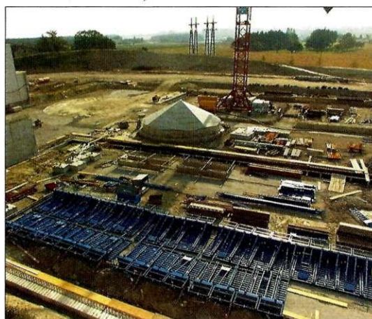
Civil engineering work on CERN's LHC collider is already underway on Swiss territory.
